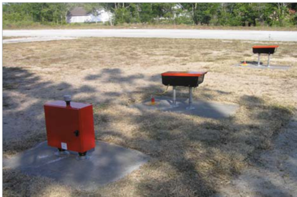
Fig. 2 Typical Installation of a PAPI A Light Unit
