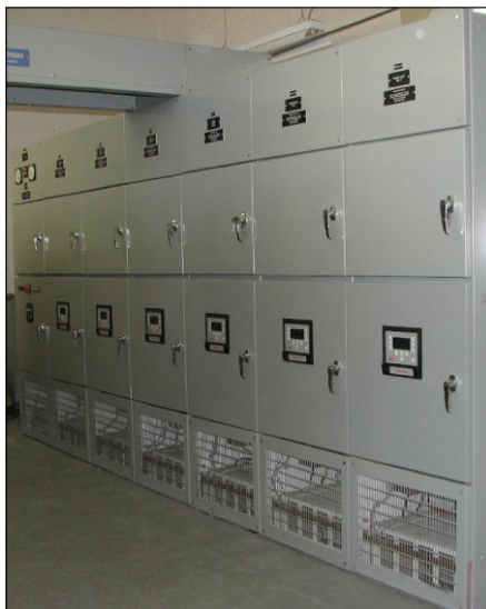
2400V Liberty Digital Switchgear regulators installed next to existing RSS20 CCR. Cell dimensions are 1" w × 1" h × 31.1" d.
