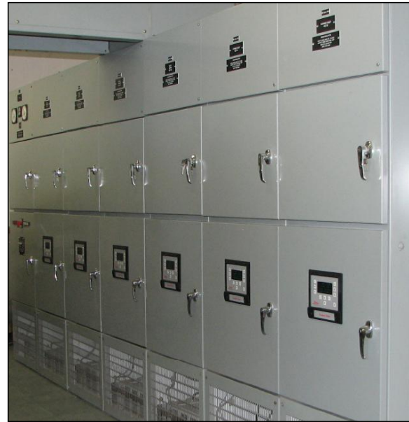
Fig. 1 Liberty 2400V CCRs installed next to RSS20 CCR.
